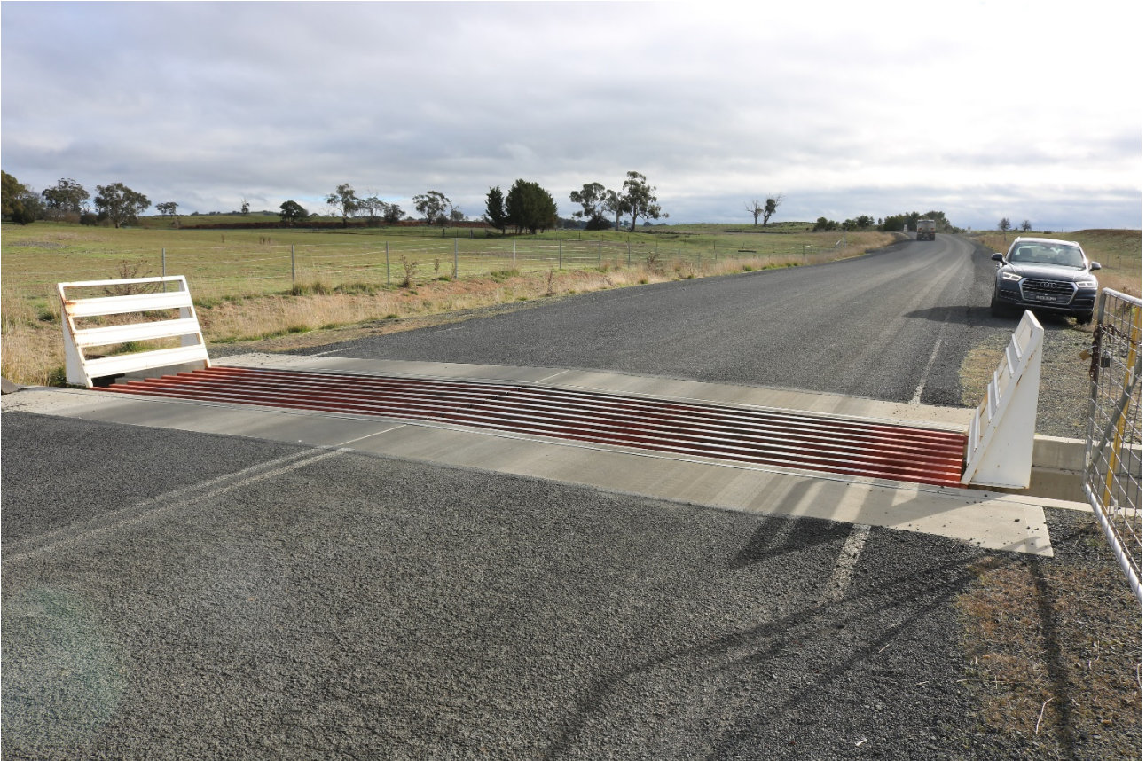
Photograph 2 – Shaker Grid at Quarry entrance
