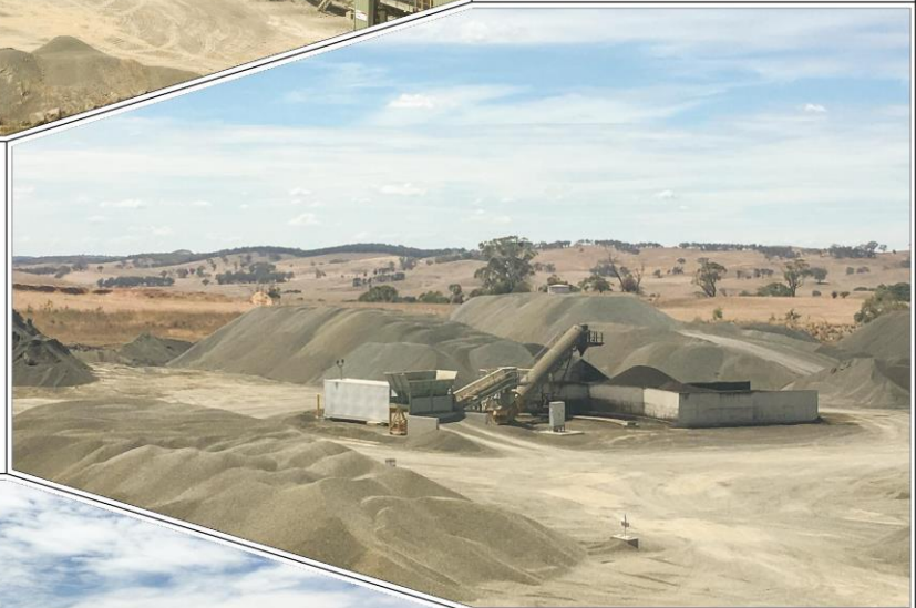
Plate 10: View of the northern section of the Infrastructure Area including the Pre-Coat Plant and various aggregate stockpiles (Ref: Plate 10)
