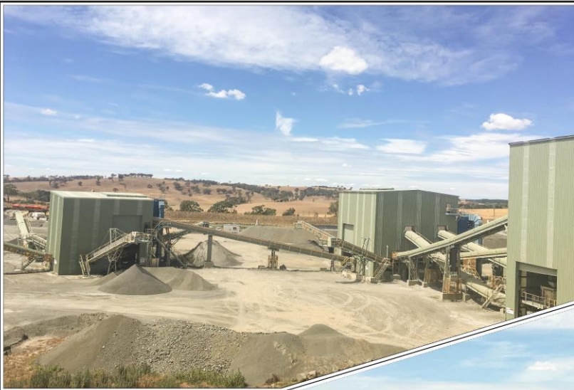
Plate 9: View of the southern section of the Infrastructure Area including the Fixed Processing Plant (Ref: Plate 9)
