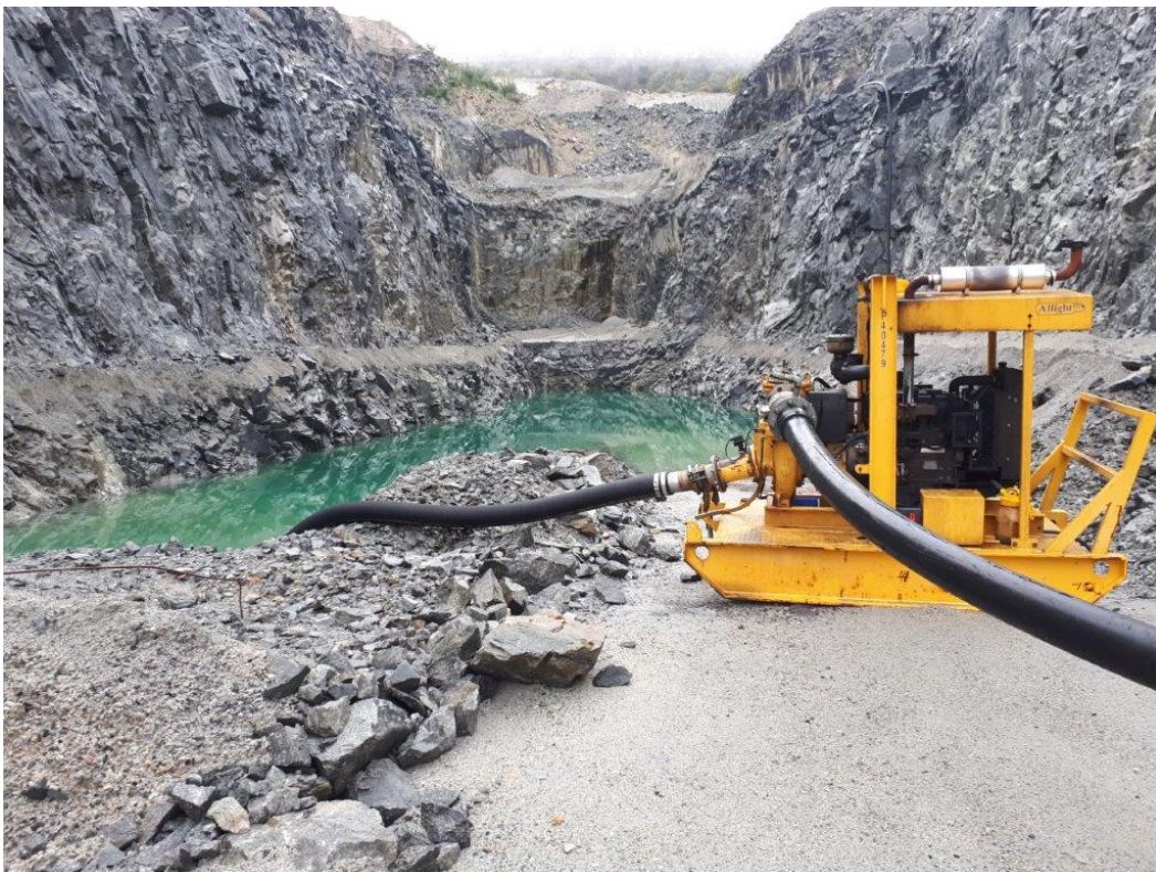
Plate L Pit base and pump
