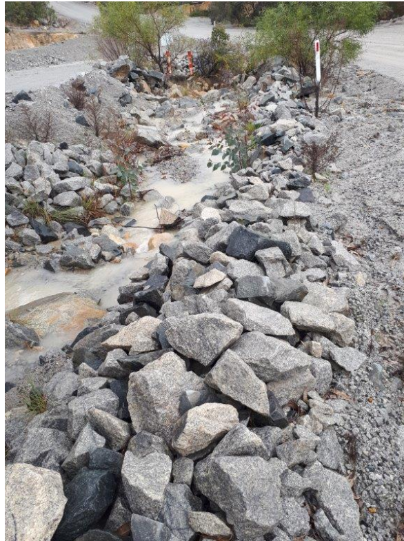
Plate I Drainage channel along main haul road
