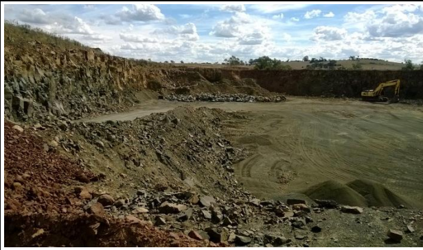
Plate 9 View of the southern and western faces of the Extraction Area facing west (Ref: E869G_008)
